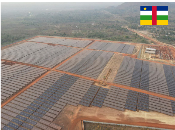
SolarTerrace MAC Central African Republic 25MW
